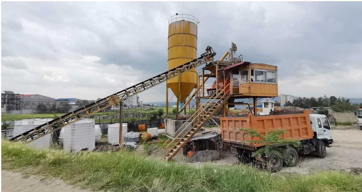
Concrete Batching Plant
